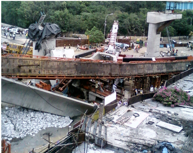
Delhi Metro Rail Construction disaster that claimed six worker's lives.
